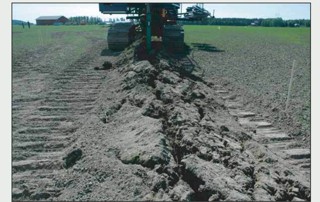
Drainage plow was used in this method. The trench closes right after the pipe laying.
