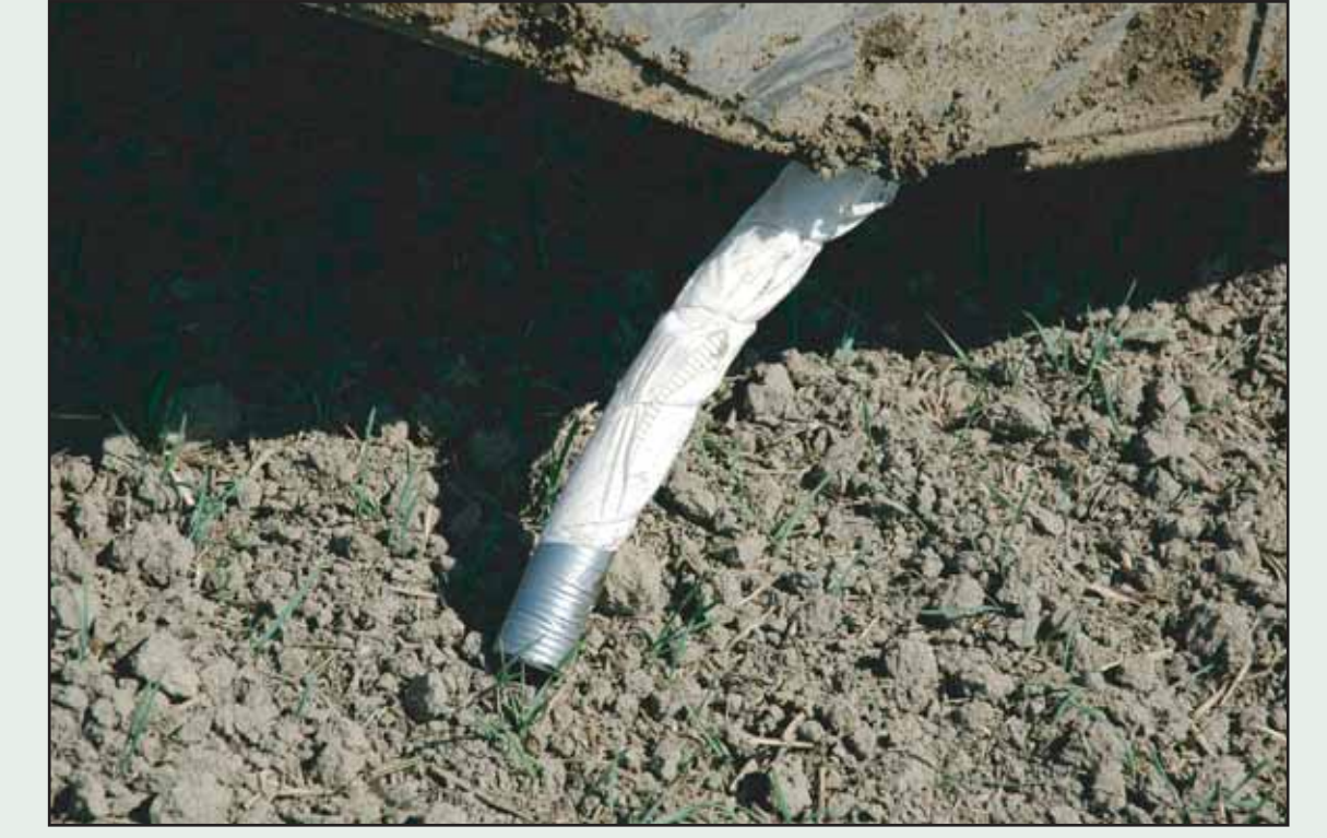
In method II a very thin textile (<1 mm) was used as an envelope. Drain spacing was 6 m. The old pipes were destroyed.
